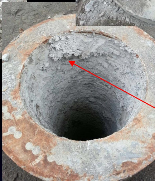
樁頭端部—樁內壁髒污，樁芯日後摩擦力大降
